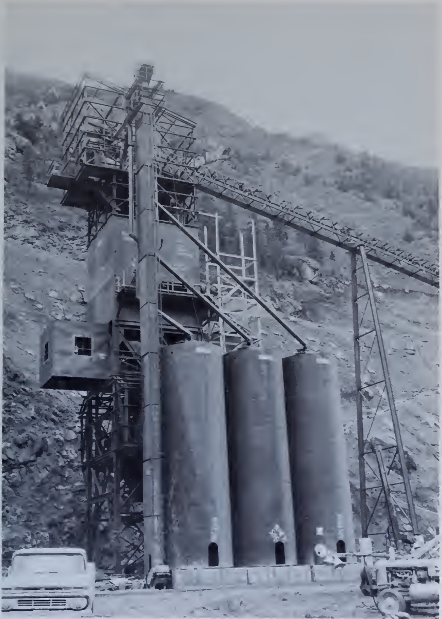
Figure 93.—Concrete batching and mixing plant at Morrow Point Dam in Colorado. P622B-427-2945.
